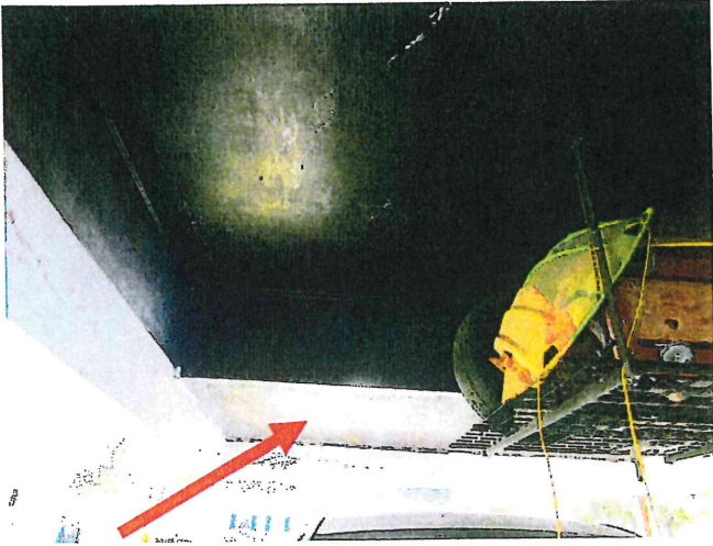
Photo 1: Carport Lower Ceiling
